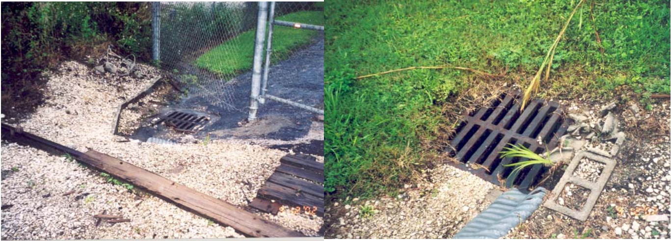
Photograph 12 & 13: Storm water grates leading to surface water drainage system, left photo outside of property, right photo inside of property.
