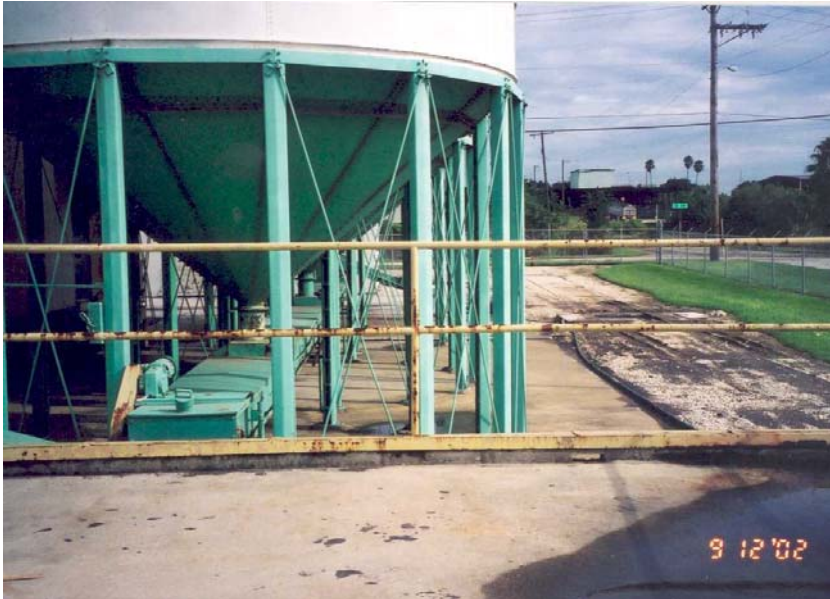
Photograph 10: Storage silo on the east side of the building, looking north from the loading dock.
