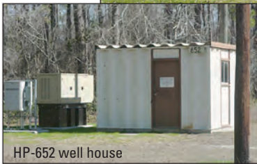
Hadnot Point water treatment plant (Building 20)
